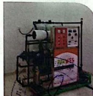
REVERSE OSMOSIS PLANT
